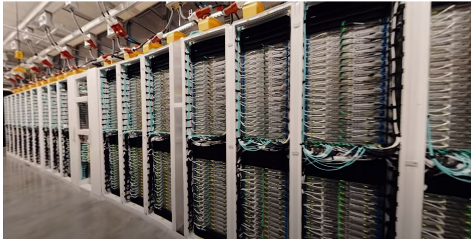
Partial View [4] of an aisle in a Microsoft Azure Datacentre
